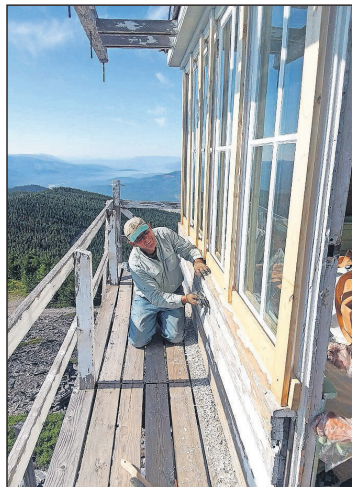
THE NORTHWEST Montana Chapter of the Forest Fire Lookout Association has done a number of projects this summer, including repainting the exterior of the Mount Brown Lookout in Glacier National Park. (photo provided)
