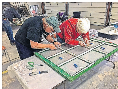
MARK AND Karen Sheets refurbish original windows from the Mount Wam Lookout in the Kootenai National Forest. (photo provided)
