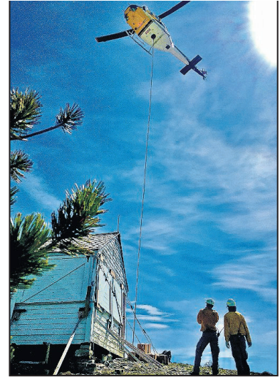
MATERIALS FOR restoration projects are carried to fire lookout sites via pack animal or helicopter. (photo provided)
